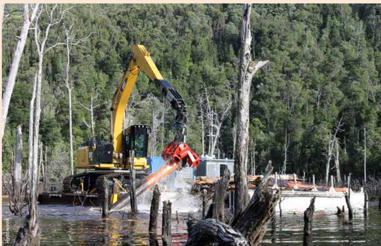
Hydrowood purpose-built, waterproof harvesting head and boom attached to an excavator mounted on a barge.
